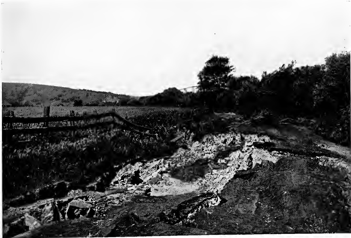
B. Destruction of road due to lurching of ground toward Salinas River. Near Spreckels. A. C. L.
